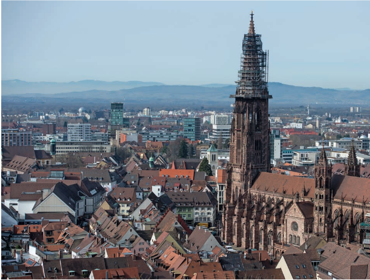
The Gothic spire of Freiburg's cathedral, being refurbished here in February 2014, towers over the city's modern and medieval quarters.
